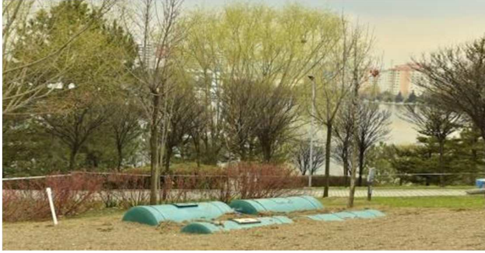
Figure 3. Rainwater Harvesting Tank in the park
